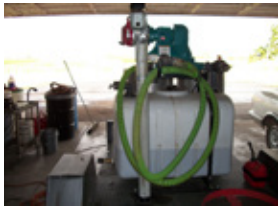
Waste oil skid mounted pump
