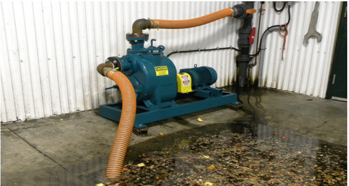
FOOD PROCESSING PUMPS Shown Trash Flow TFCC-3 installed at a Massachusetts food processing facility. End user pumps apple cores, skins and other solids. Close coupled direct drive model shown.
