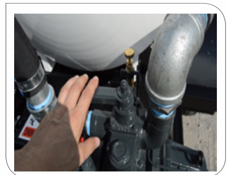
Gas, Diesel or Electric Pump Systems
