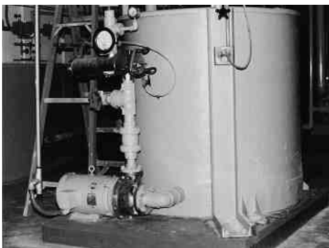
Reverse osmosis, Ósmosis invertida
